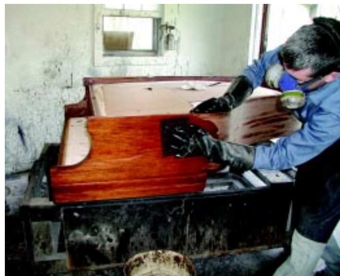
Photo 8 — The residue left by the stripper can be removed with lacquer thinner and a Scotchbrite pad.
